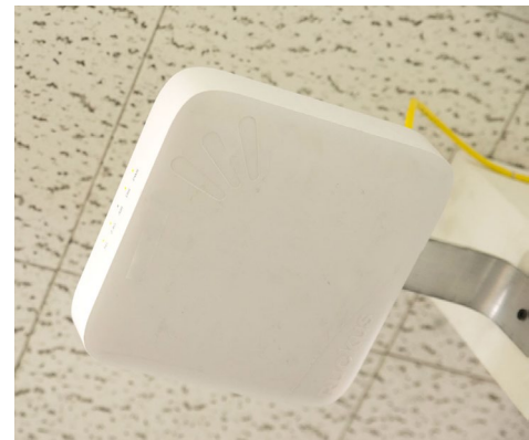
BELOW: 802.11n and 802.11ac APs are mounted dome-down with standard 802.3af PoE connections.
