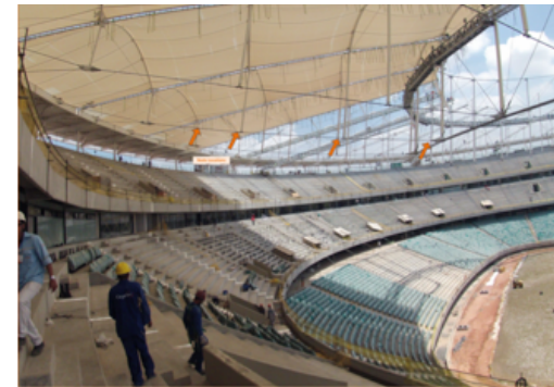
Figure 2: (Above) Arena Fonte Nova in Brazil with 151 Ruckus Wi-Fi APs during construction
